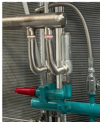
Safety valves on HP side (set 25 bar)
