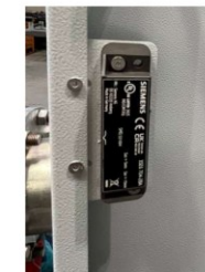
Safety switch on the back door to switch off the unit
